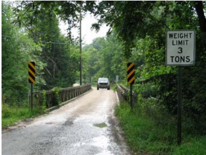
(Above) The existing Wilbur Road Bridge carries a weight restriction of 3 tons - the minimal weight restriction allowed.
