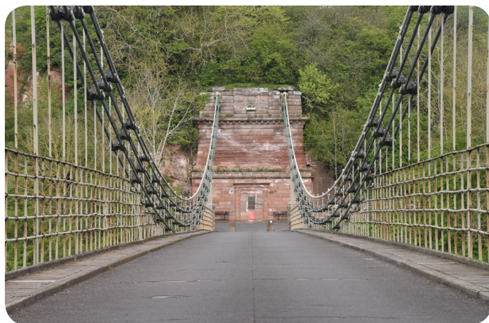
A view on bridge facing toward England (east). Photo by Nathan Holth.
