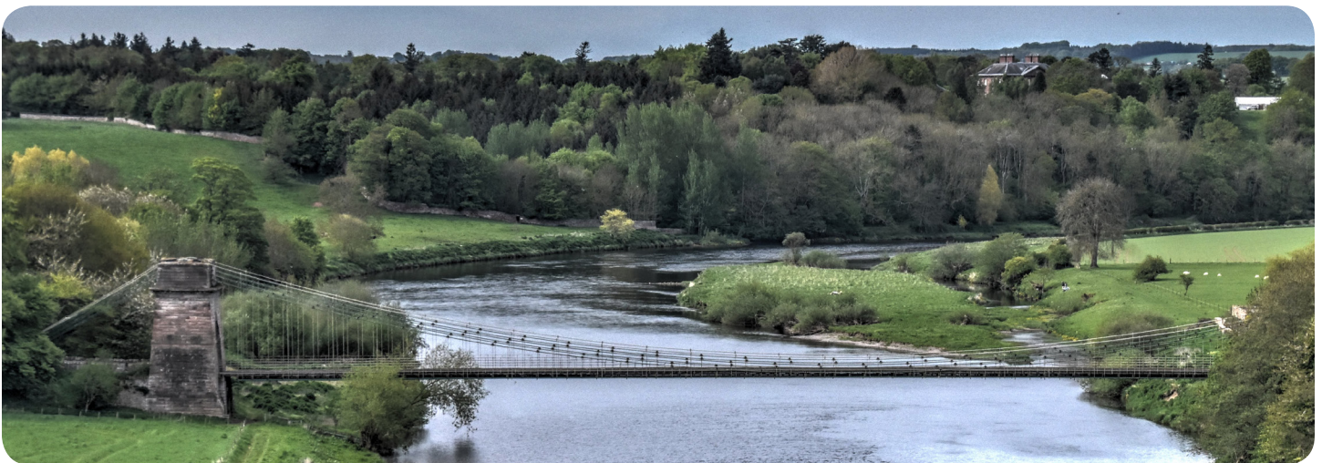
South elevation of the Union Chain Bridge. Note the asymmetrical layout of the main eyebar chain system, since the west (left) end has a tower and anchorage, while the east (right) end has only an anchorage, and at that end the eyebar chains do not rise to the same elevation as the end with the tower. Photo by Nathan Holth.
