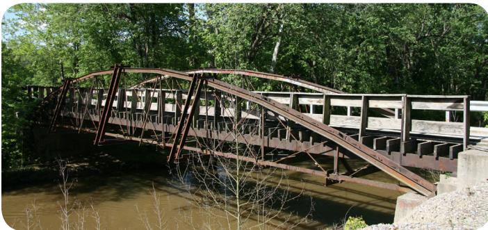
View illustrating the arched top chord of the bridge. Photo by Nathan Holth.
