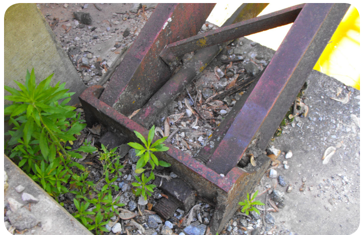
Detail of bridge shoe where top and lower chords meet. Photo by Nathan Holth.
