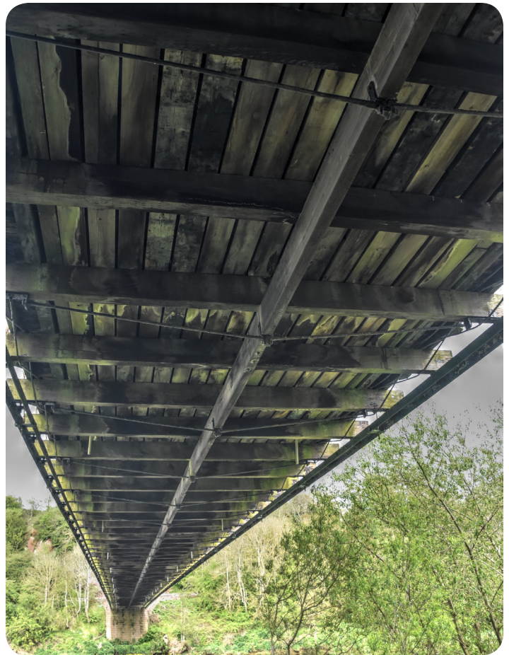
This photo shows the timber decking and floorbeams of the bridge. The floorbeams also include metal tension rods. Photo by Nathan Holth
