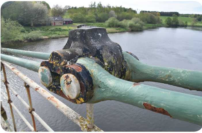
Detail showing the original loop-forged eyebar chains and the two-pin cast iron connectors that were typical of early eyebar chain suspension bridges. Photo by Nathan Holth.
