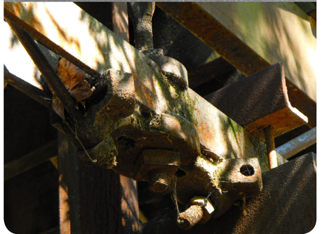
Top: Upper end of diagonals. Bottom: Lower end of diagonals. Photos by Nathan Holth.
