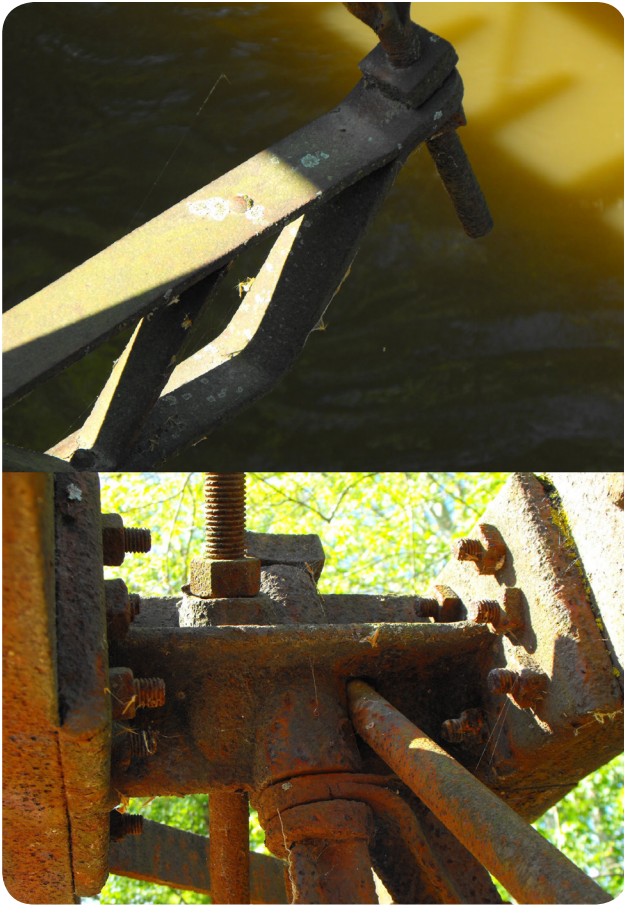
Details of the sway bracing connections on the bridge. Photos by Nathan Holth.
