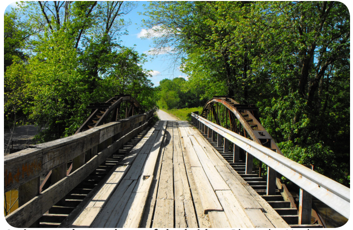
A view on the roadway of the bridge. Photo by Nathan Holth.
