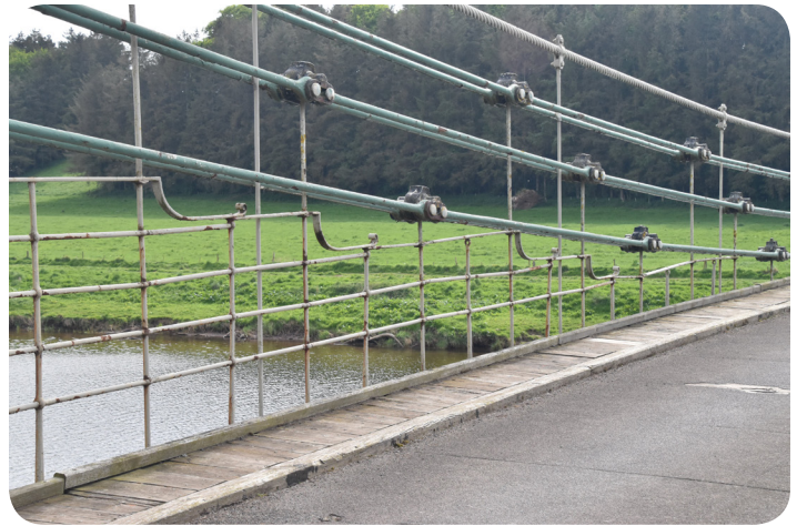
View on the bridge showing the 1902 wire cable on the top, the three rows of original paired eyebar chains below, and at the bottom the railing which is carefully designed to fill in the changing gap between the chains and the roadway. Forged openings in the horizontal railing rods allow the vertical rods to pass through. Photo by Nathan Holth.
