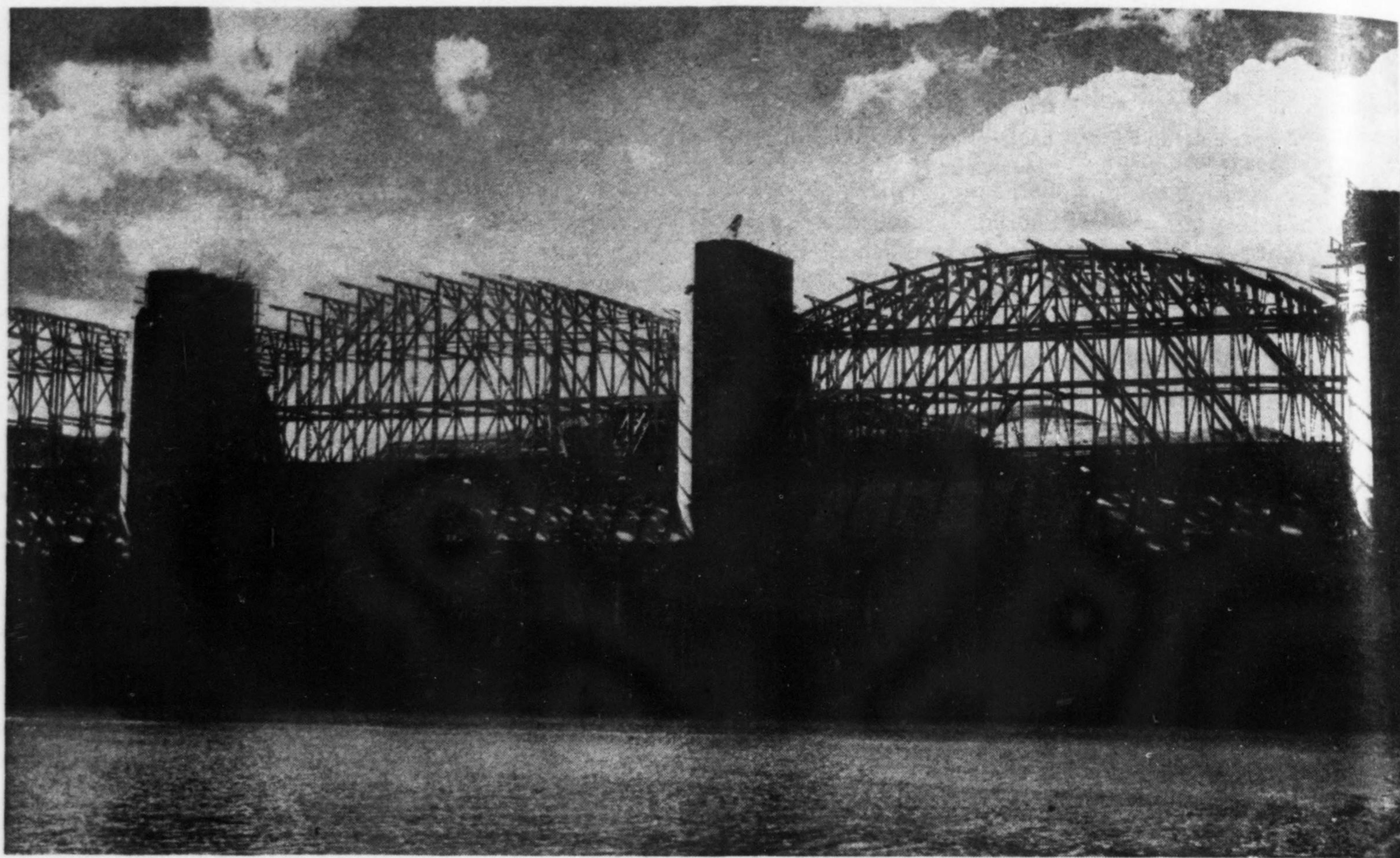
Falsework for highway bridge arches across Grand Coulee Dam spillway. The eleven spans were formed at one time.
