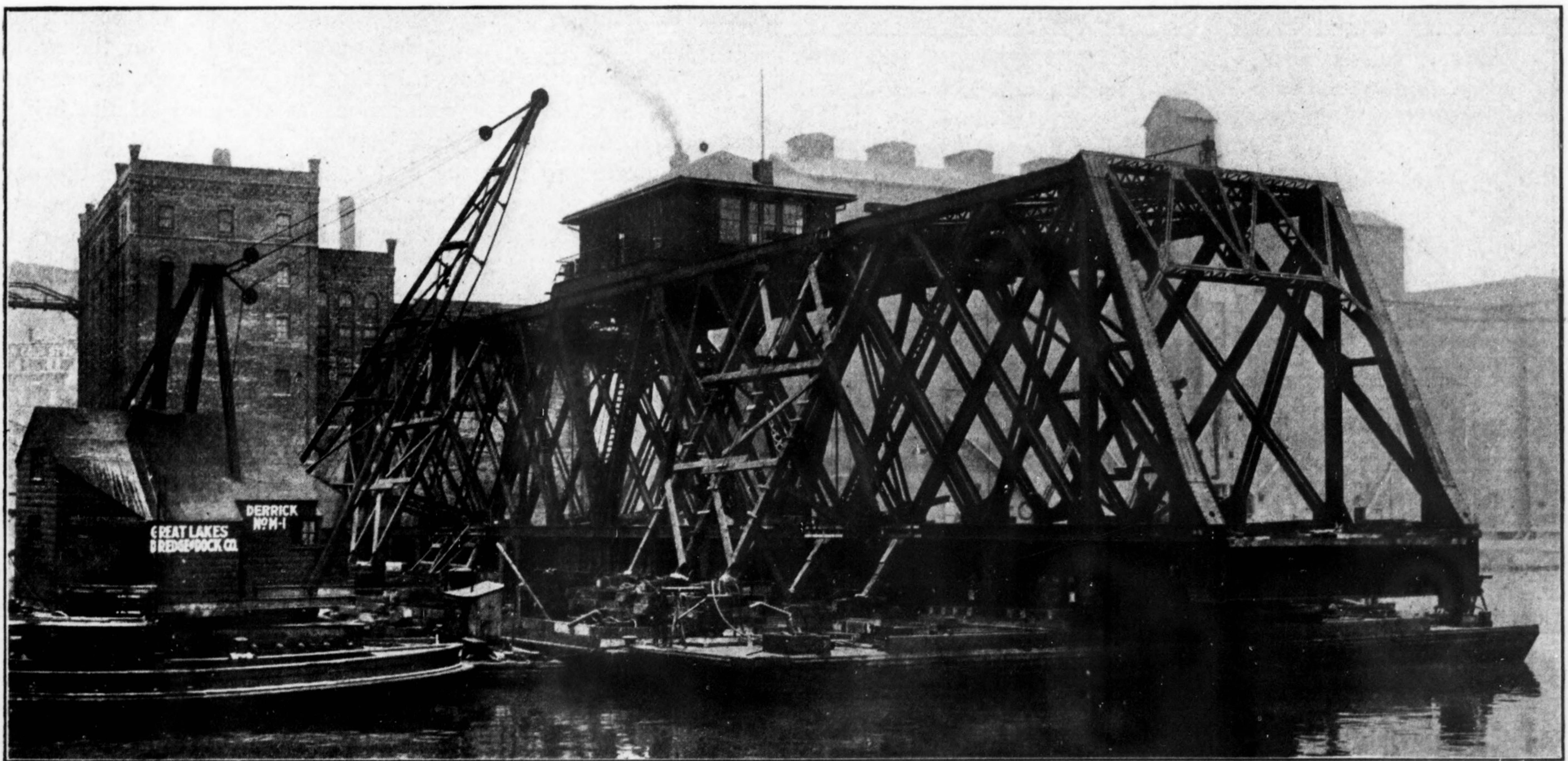
Floating the Milwaukee River Bridge on Four Scows Showing Diagonal Bracing for Distributing Loads on Two Main Scows
